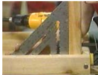
Use both a square and a clamp to hold the leg while installing the screws
